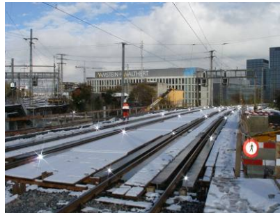
■ Monitoring prisms on the temporary bridge for deformation tracking.
