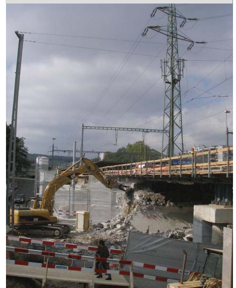
During digging off parts of the fundament of the power line pylon it was automatically measured to detect 3D deformations and the resulting change in tilt.
